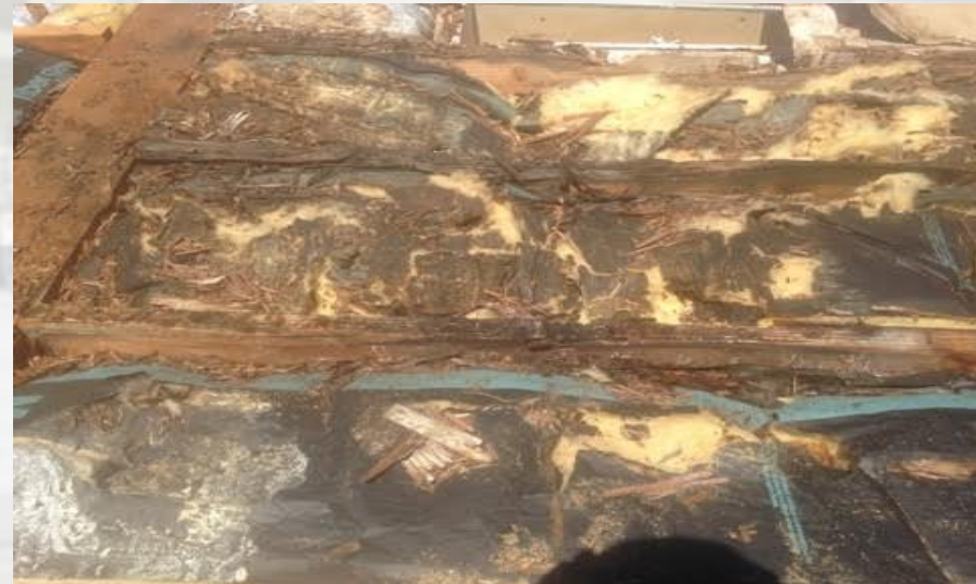
DAMAGED PURLINS ATTACHED TO ROOF TRUSSES
